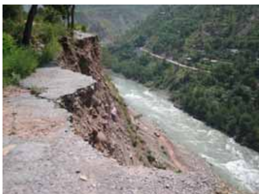
Landslides can cause roads to be cut off completely. Photo: UNJLC.
