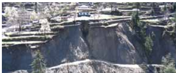
Many roads in the Earthquake affected area are at risk of further landslides during the Monsoon season.
